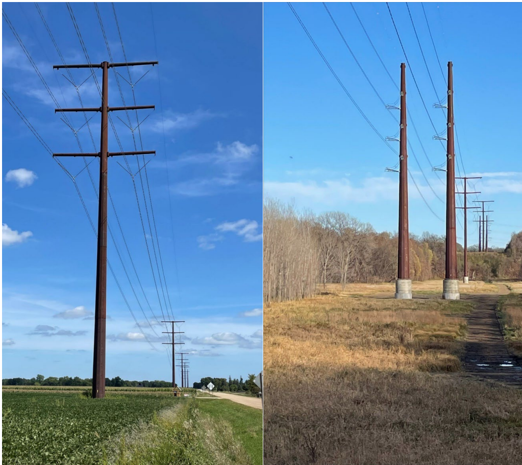
Typical Double Circuit Structures | Typical Dead-end Structures
